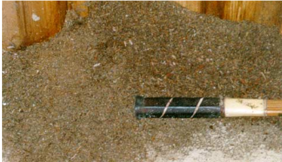
Evidence of carpenter ant activity.
