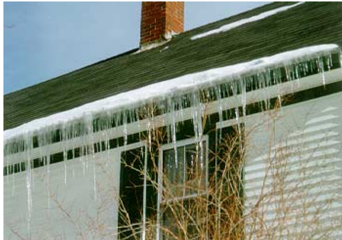
Icicles may indicate inadequate attic insulation or limited attic ventilation.
